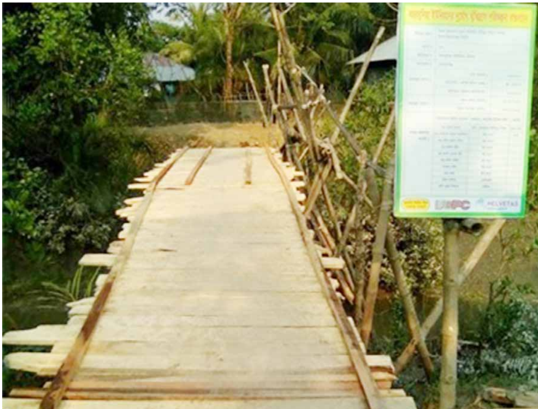
A 'wooden bridge/culvert' constructed jointly by the Local Government Institution, NGOs and Local Community in Godaipur village at Paikgacha upazilla in Khulna district. It is one of the examples of the implementation of the RRAP by collaborative and joint action at the local level
