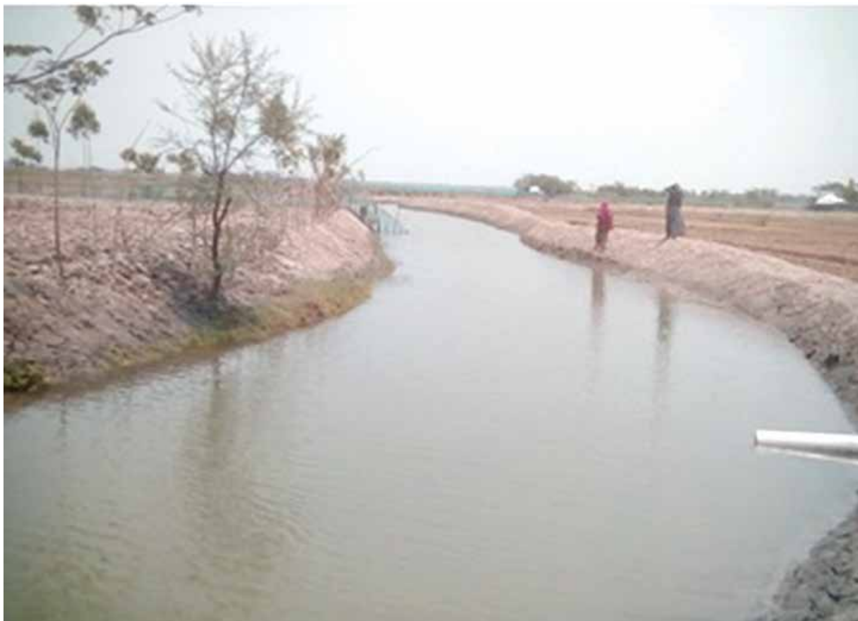
Goroikhali-Gangrothi embankment at Goroikhali union in Paikgacha upazilla, Khulna district, an example of joint initiatives through influencing and resource mobilization
