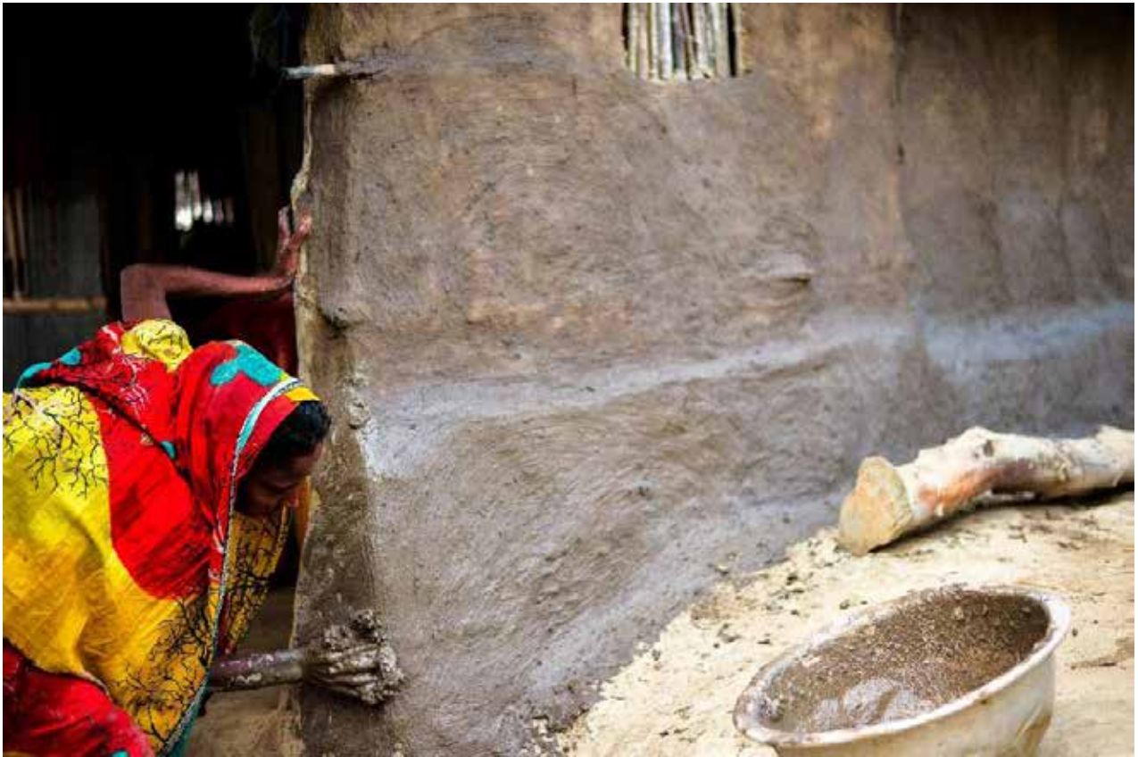
Rabeya Khatun, living in the outskirts of Sundarban in Shyamnagar explains, "I need to re-apply the mud paste every 5 days over the outer surface of my walls, otherwise the mud plaster crumbles and breaks down. It is a very tedious process. Today I am very sick, but I still need to get this job done." S ANWAR
