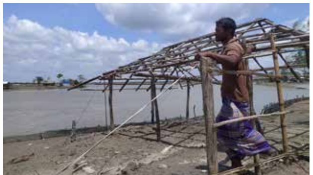
The man in the picture from Gabura is building his house again, which is right beside the river. Every year he has to rebuild the house because it gets damaged in cyclones.
