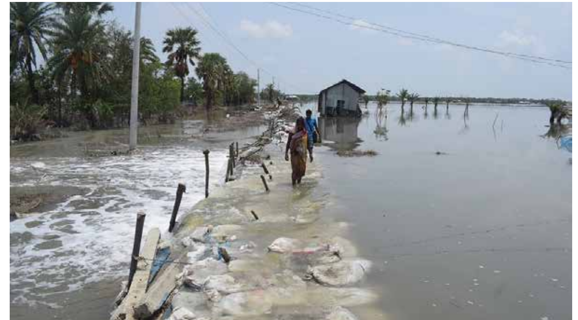
Weak embankment on the banks of the river Kopotaksh. The weak embankment collapsed due to the impact of Cyclone Amphan. The photo was taken from Hajatkhali village in Koyra upazila of Khulna district on the west coast of Bangladesh
