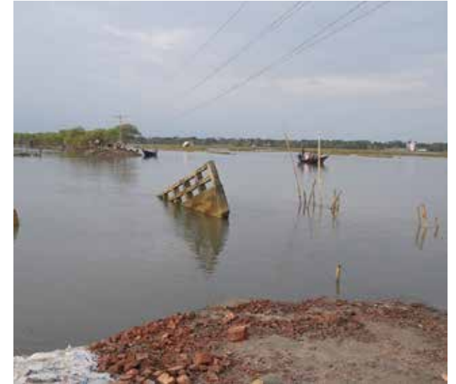
It is not a river. There used to be paved roads here. There was a culvert on that street. The culvert has collapsed under strong tidal pressure for the cyclone. The photo was taken from Fultala village in Asashuni upazila of Satkhira district on the west coast of Bangladesh
