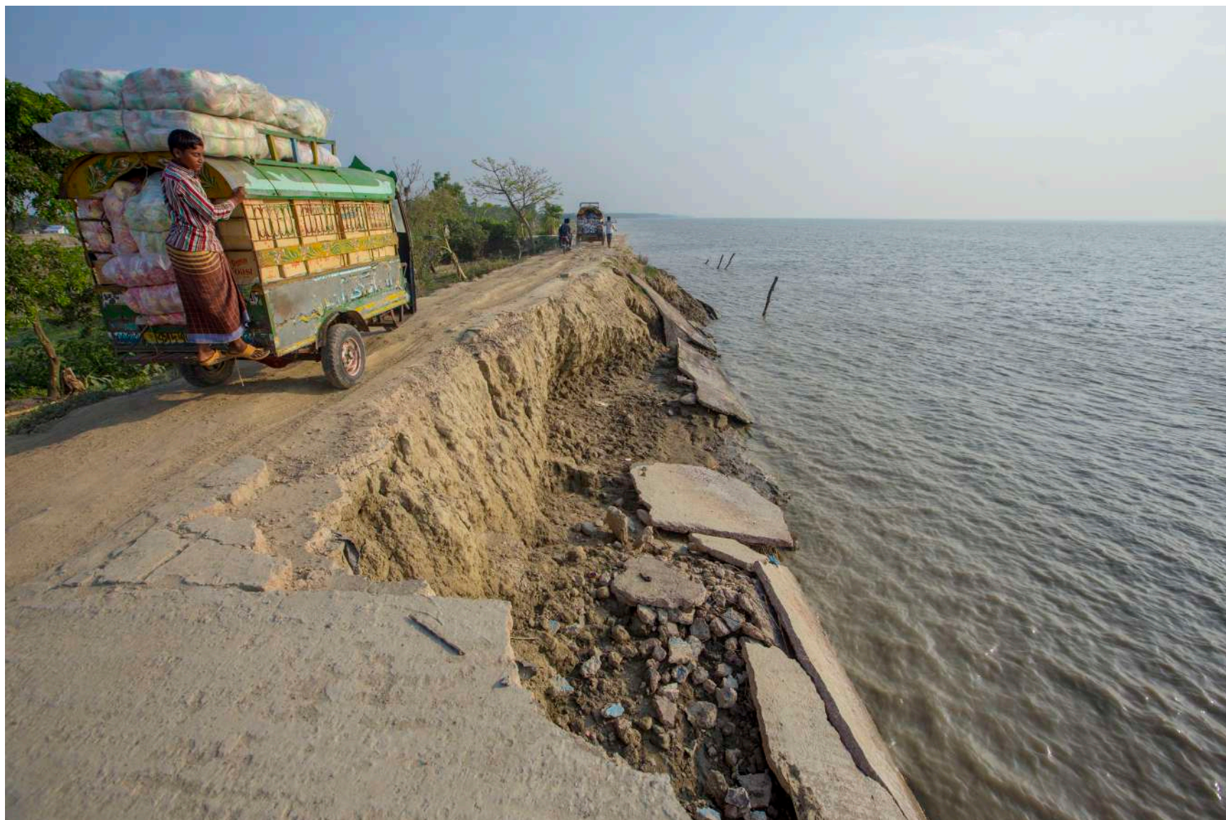
Damaged embankments in Bhola district.
